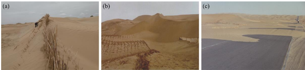
Fig. 2 Damage conditions of the mechanical sand control system caused by wind-blown sand along the Taklimakan Desert Highway. (a), buried sand barrier fences; (b), sand aggregation in the straw checkerboard barriers; (c), moving dune coverage on the desert highway.
